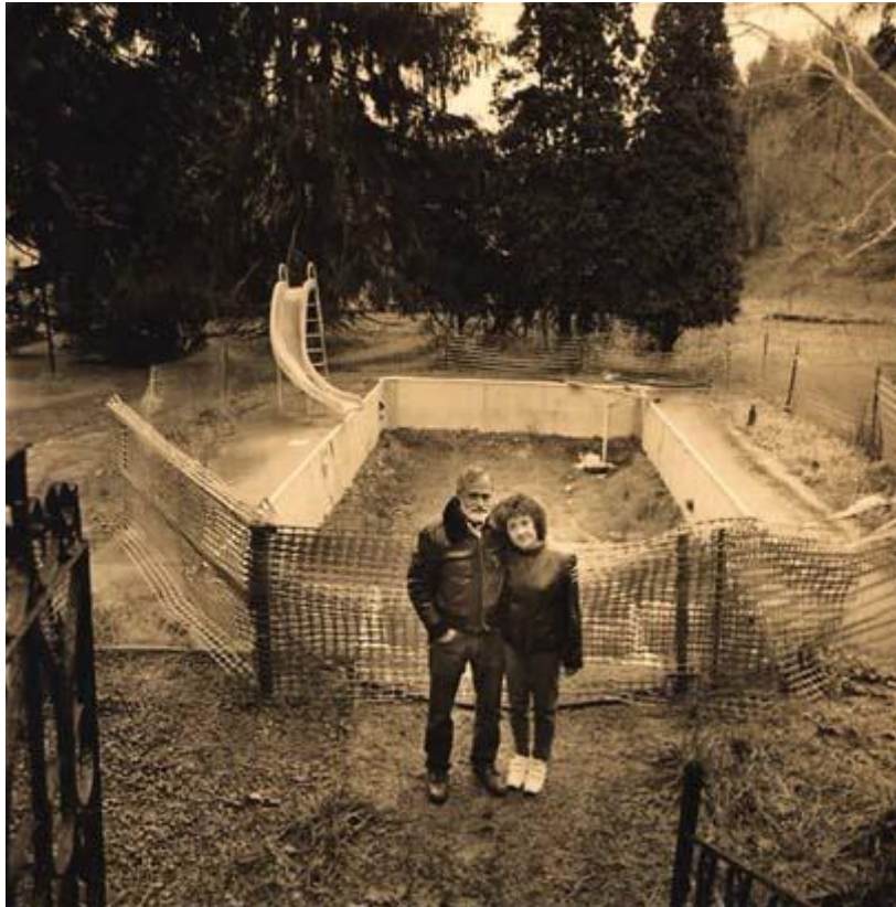
Roy and Diane Brendel in front of the undermined pool outside their Spanish Revival mansion in southwestern Pennsylvania.
